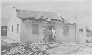
A new roof solves a big problem. Un dak nobo ta resolve un problema grandi.
